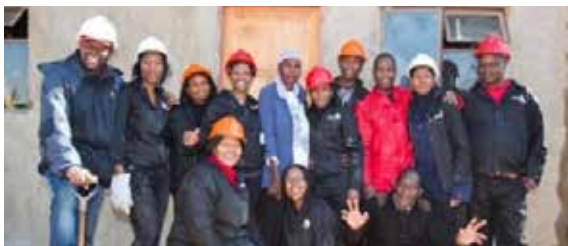
Sasria staff members volunteered their time and, together with other industry partners, helped to build two houses in Delmas
