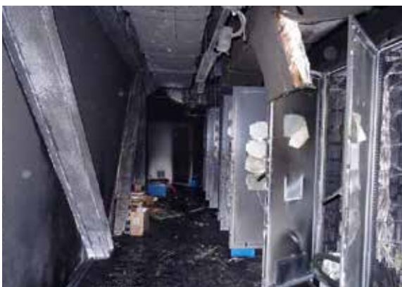
The generator control cabinets at the power plant were destroyed by the fire set by employees on strike during August 2015.
